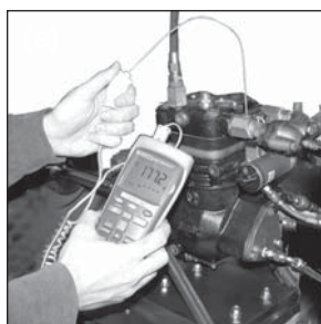
Testing the temperature at the discharge fitting.
